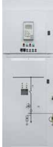
Figure 1. Front view of the switchgear
