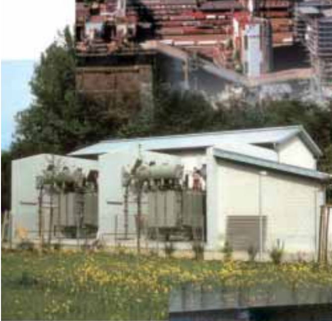
Application Public power supply system
