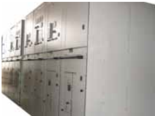
Switchgear in marine industry
