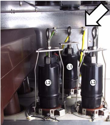
Fig. 22: Cable routing to the rear
