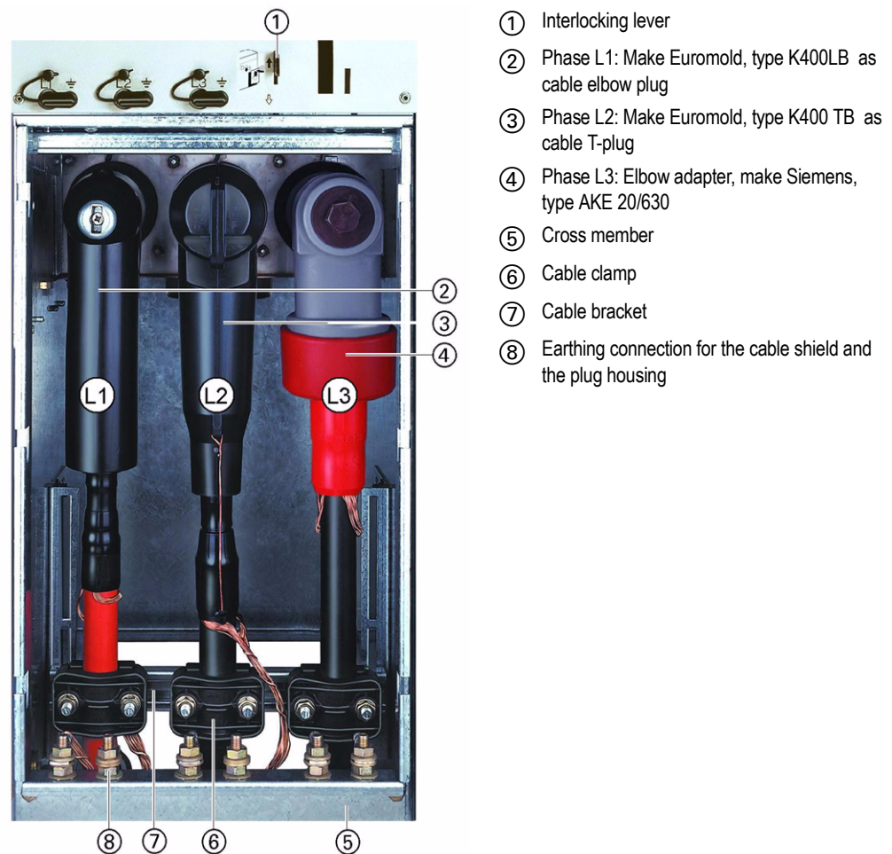
Fig. 20: Ring-main cable connection
