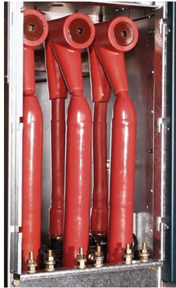
Fig. 25: Cable plug make Raychem RICS 5xxx with surge arrester type RDA 24
