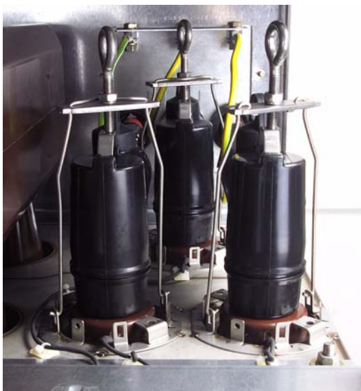
Fig. 8: 8DJ10 with transformer cable routing to the rear (make Euromold, type K158LR)
